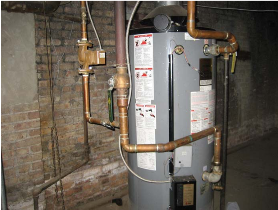
View of the hot water heater
