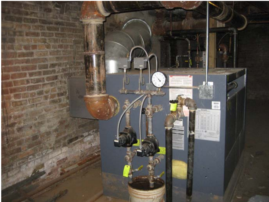
View of the boiler
