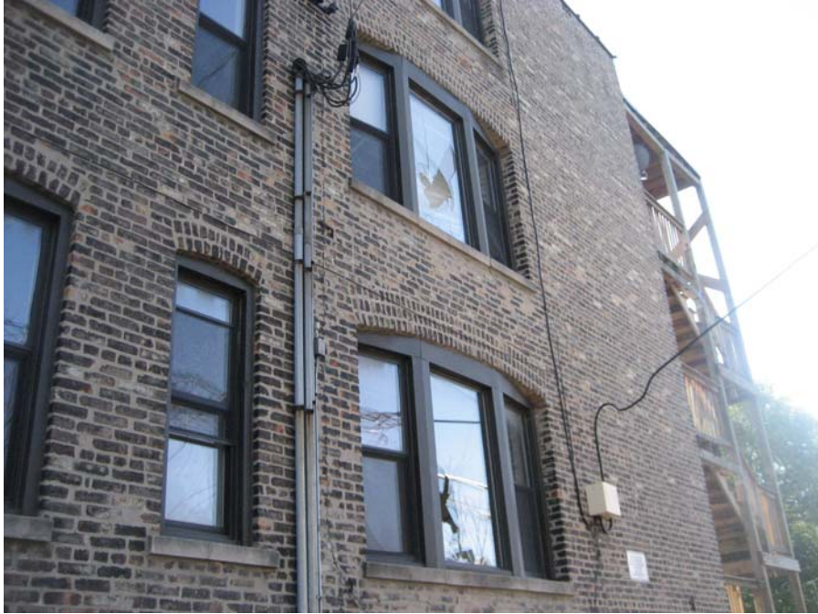
View of the subject exterior deferred maintenance
